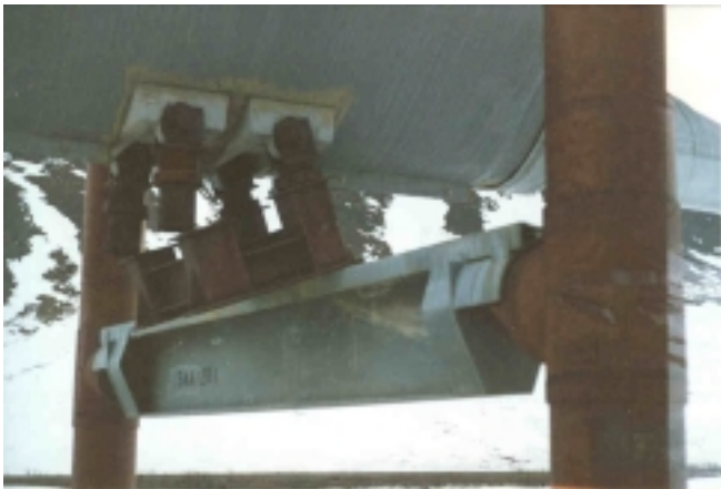
A pipeline shoe that slipped off the crossbeam during the shift. For more dramatic photos of this event, turn to pages 6-7.
