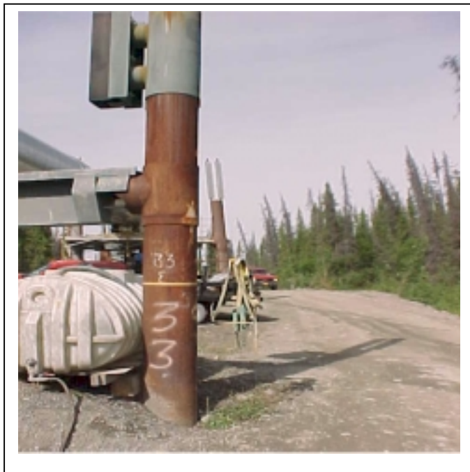
This VSM, labeled number 33, is leaning slightly to the right of vertical, while the VSM behind it is leaning to the left of vertical.
